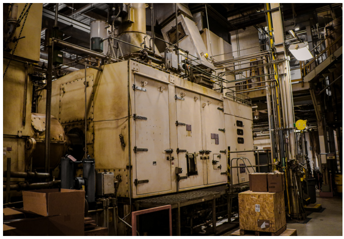
A General Electric LM-1600 aeroderivative turbine is encased in a grey steel box at the heart of the cogeneration plant. The turbine was modified from the General Electric F404 aircraft engine series, which powers the F/A-18 Hornet fighter jet. It can generate up to 15 MW of power for Princeton—enough to power a small town.
